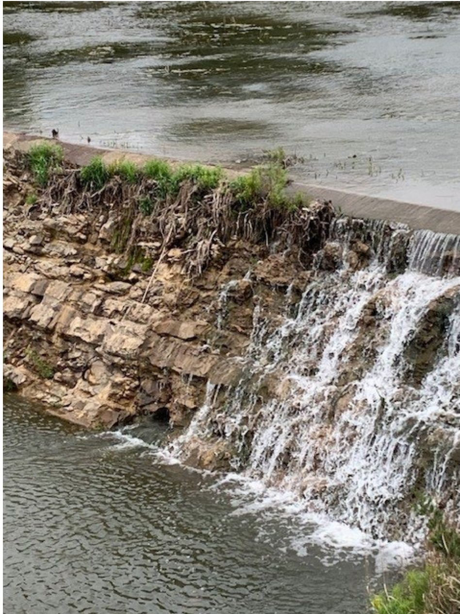
Pic. 3 – Area of concern, shown at base of of the spillway as a black “hole”; immediately left of cascading water in picture.
